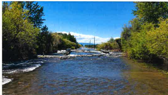
Flood event of 2017; overtopping bridge
