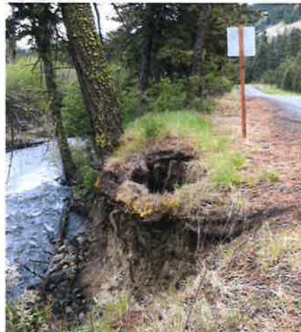
Undercutting of bank
