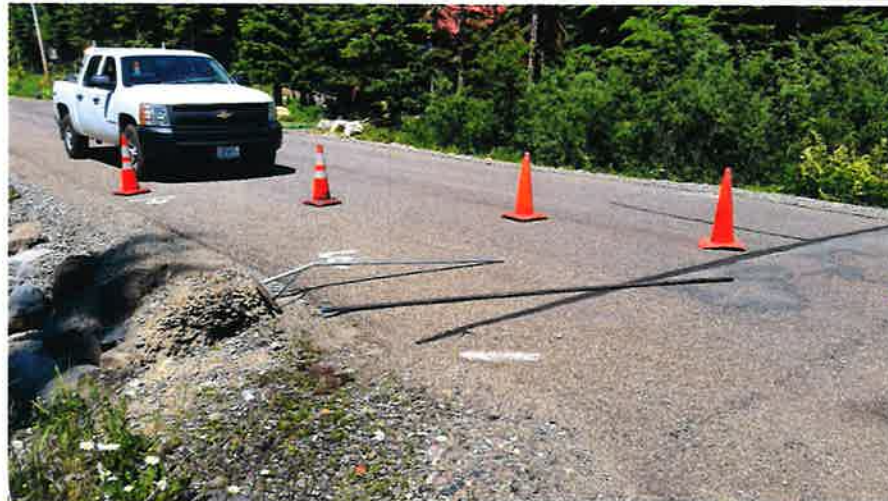
Yellowstone Rd at failing culvert
