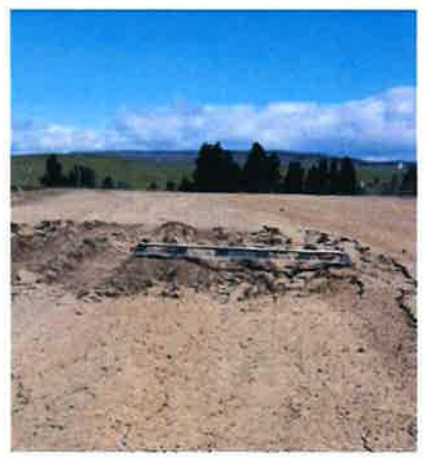
Horlick Rd damage from heavy truck traffic
