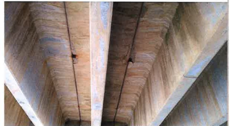
Spalling at weld tabs
